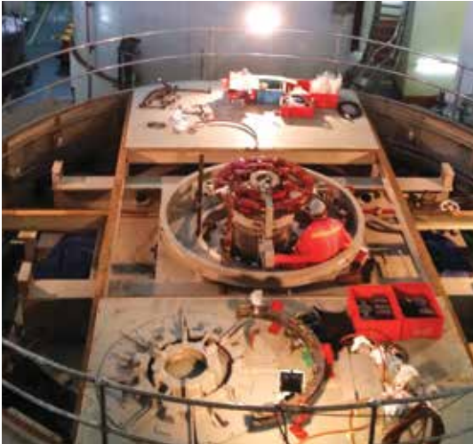
Hydro turbine electro-hydraulic governor (load/frequency) control system for SJ Tenom Pangli, Sabah
