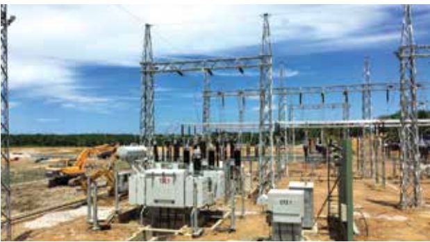
132/33/11kV power distribution system for Sakura Ferroalloys Project
