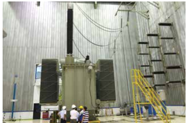
120 MVA 275/36kV Power Transformer FAT at PT CG Power Systems Indonesia
