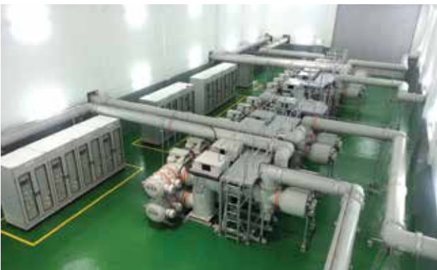
GIS (Gas Insulated Switchgear)
