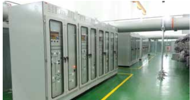
Local Control Panel (LCP) for Financial centre 132/33kV GIS Substation
