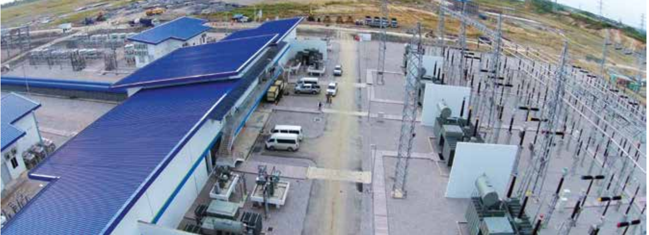
"275kV substation for the Ferro Alloy Project" of OM Material (Sarawak) Sdn Bhd
