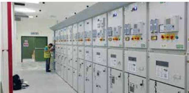
33kV Switchgear Panel for Sakura Ferroalloys Project
