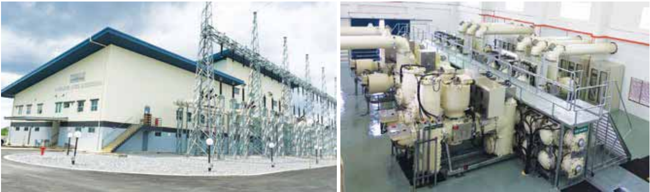
Samajaya Project - the first 132kV Gas Insulated Switchgear Substation in Kuching, Sarawak
